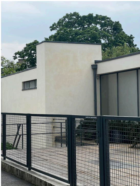
Fig. 5.03 Cloudy stains on outer surfaces of Villa Tugendhat ©Adam Hudec
